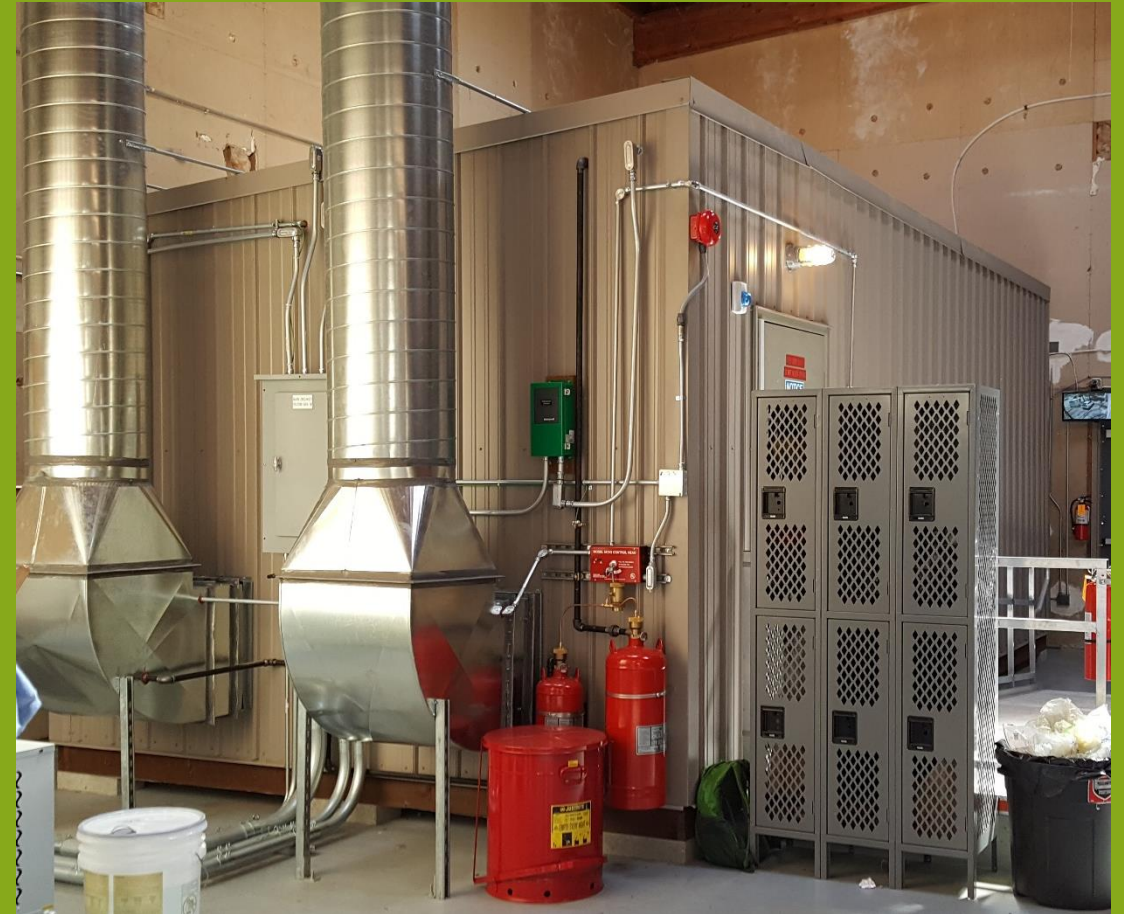
Fully Contained Hydrocarbon Extraction Unit for Cannabis Class 1, Division 1 room (which is spark free and rapidly exchanges air)
