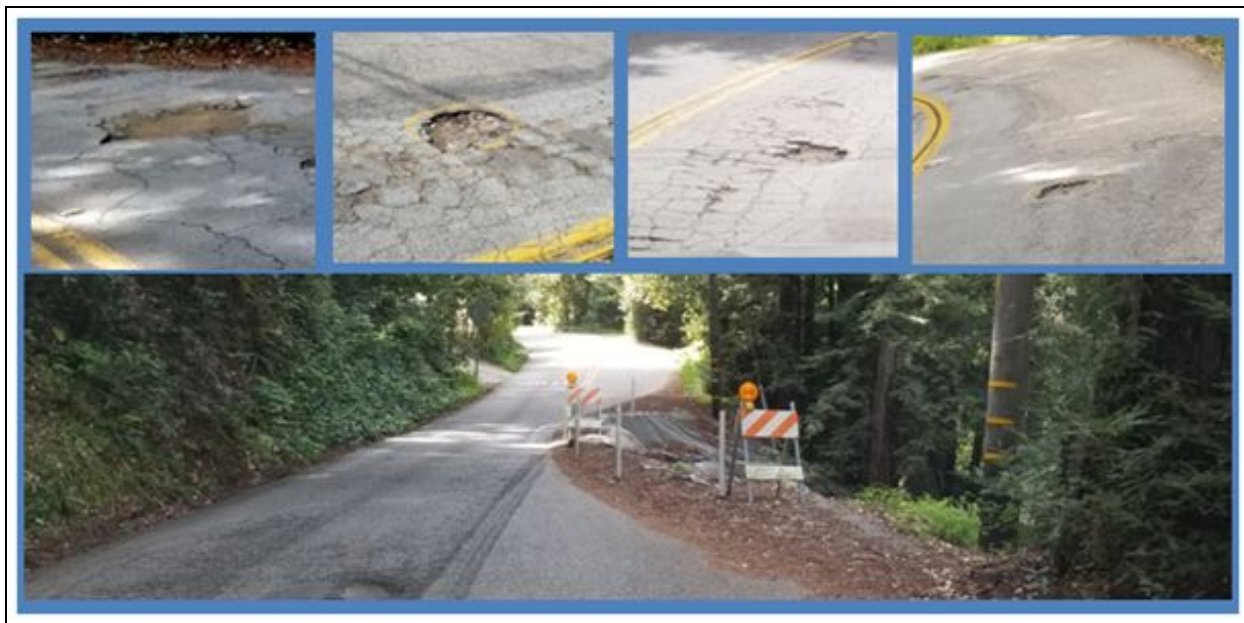
Figure 21. San Lorenzo Valley Evacuation Route - Alba Road conditions [227]
