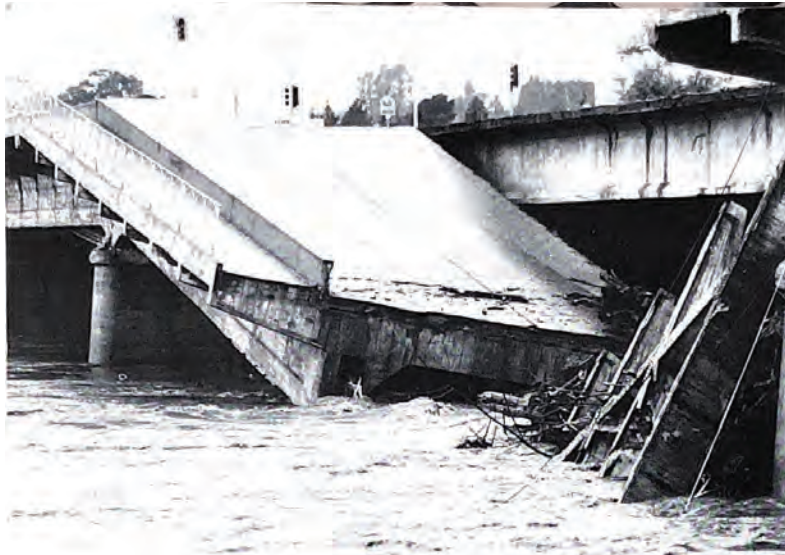
The Soquel Avenue Bridge was the raging San Lorenzo River's major victim in the city of Santa Cruz.
