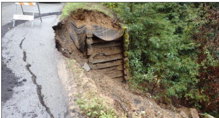
Miller Cut Off was one of several County roads damaged during March storms.
