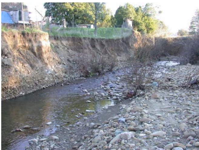
AN ERODING STREAMBANK
