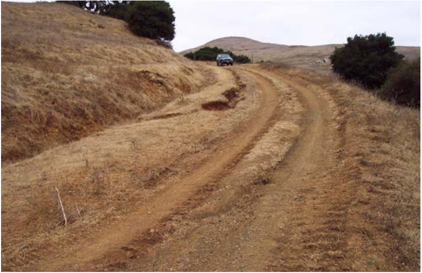
A RUTTED AND GULLIED ROAD, BEFORE TREATMENT
